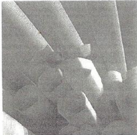
Ribbed plastic pipes stacked near a road construction site where they will be laid for drainage along the sides of a new section of motorway.
